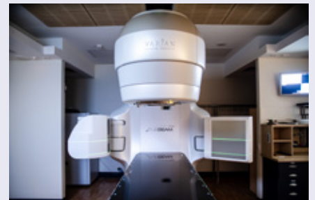
The Varian trueBEAM Linear Accelerator was installed in 2018, cutting radiation therapy treatment times in half.
